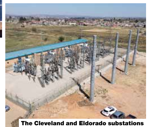
The Cleveland and Eldorado substations
