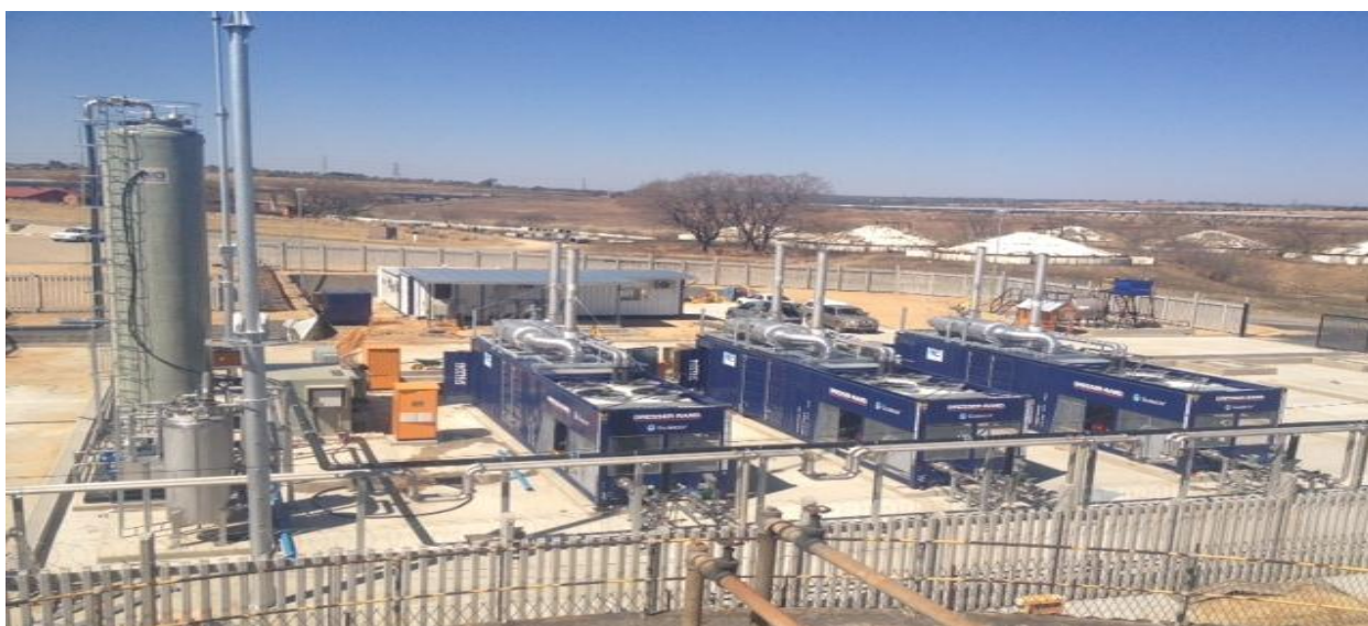
Combined Heat and Power “Biogas-to-Energy” Plant – Northern Works
