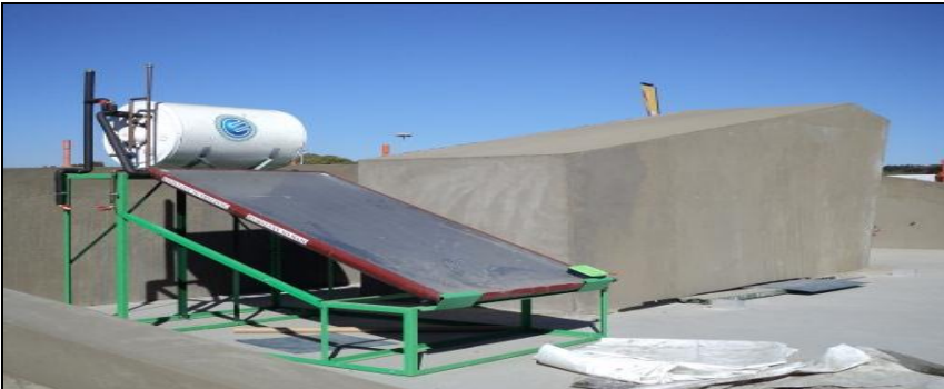
Figure 11 Energy efficient house project: Innesfree Park Sandton showing installation of solar water geysers
