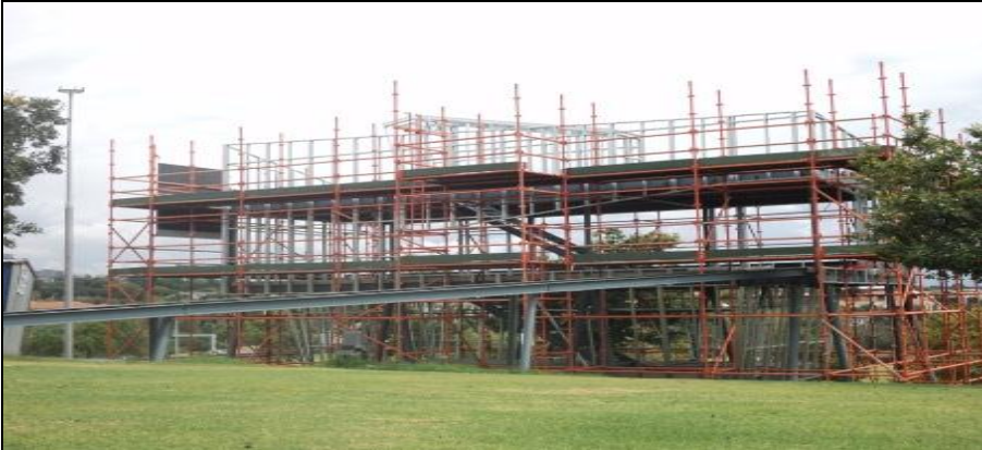
Figure 10 Energy efficient house project: Innesfree Park Sandton showing the building of the super structure
