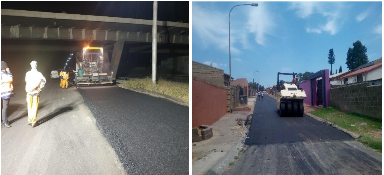
Image 1 & 2: Resurfacing of M2 Highway in Region F and Njambayi Streets in Region D
