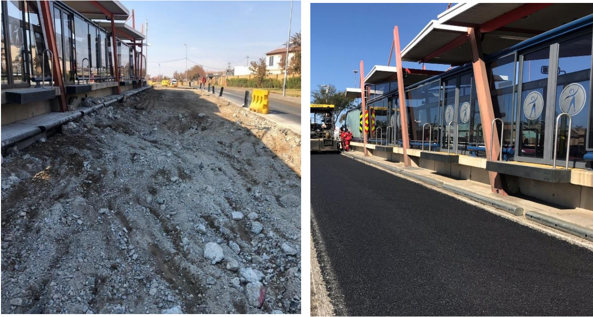
Images 7 & 8: Rehabilitation of Phase 1A and Phase 1B BRT Trunk routes and stations
